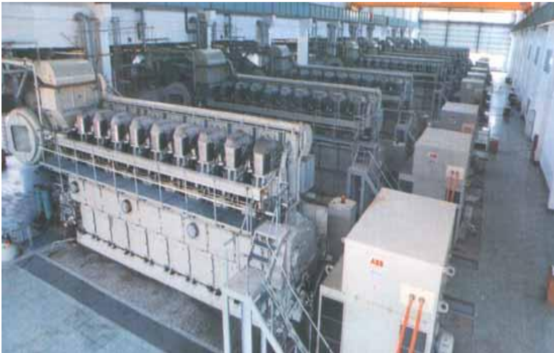
9 diesel engine power generation sets type 9TM620
