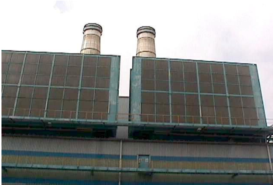
Air Filter House
