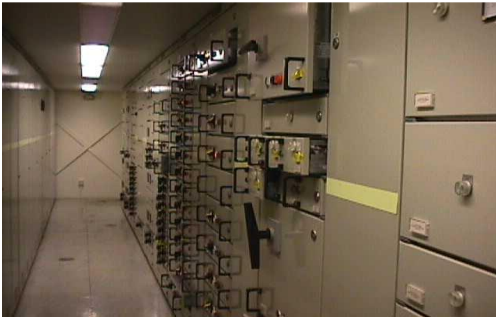
Motor Control Panel
